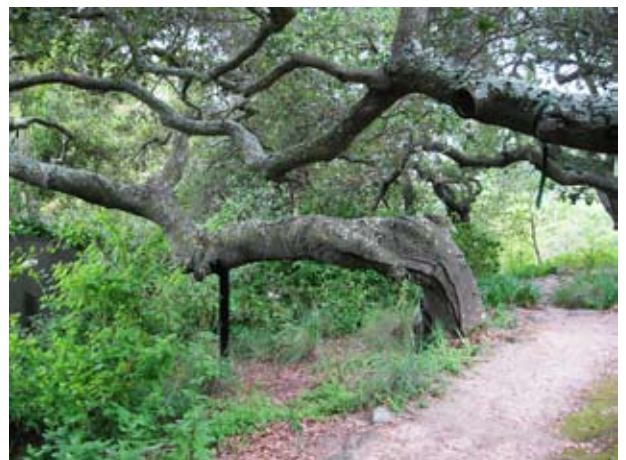
The client chose to mitigate the risk of trunk failure by having a specialized arborist install a tree prop.
